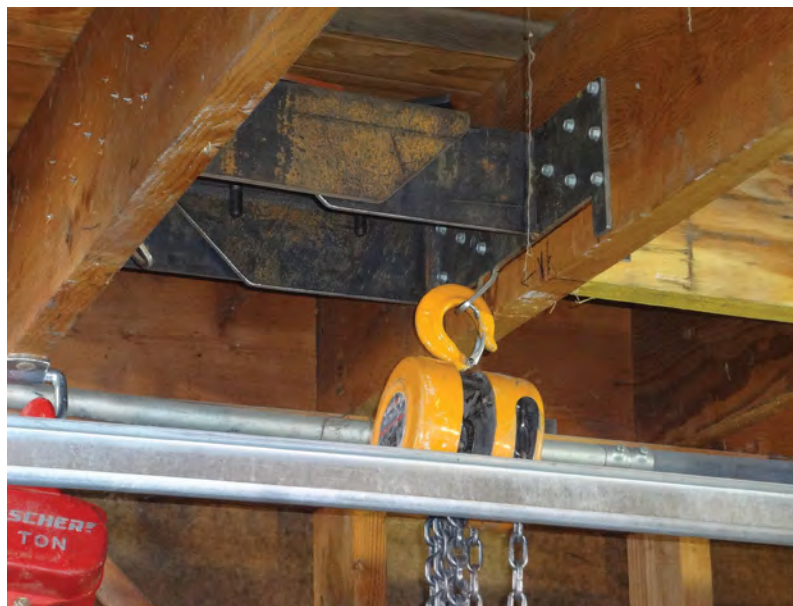
MOUNT THE BRACKETS The two manufacturer-provided brackets nest together and telescope out to fit between joists. Tabs on the brackets line up with the bottom of the joists and have holes for connector nails, which hold the brackets in place until we install the required structural screws. Placing the bolts that connect the column to the brackets through the slots in the brackets keeps the parts aligned.
